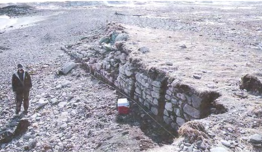
Curtain wall exposed in February storm
